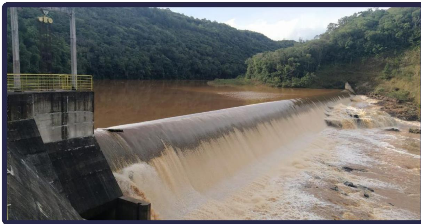
PCH Santa Carolina
